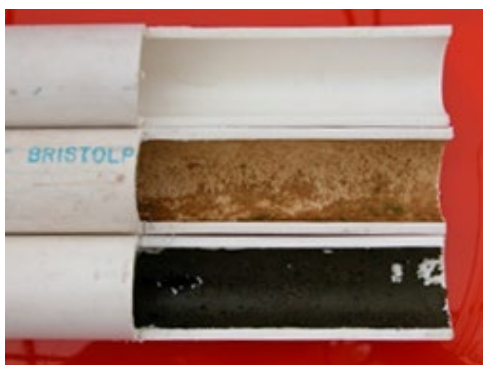
Examples of biofilm formation in pipework
